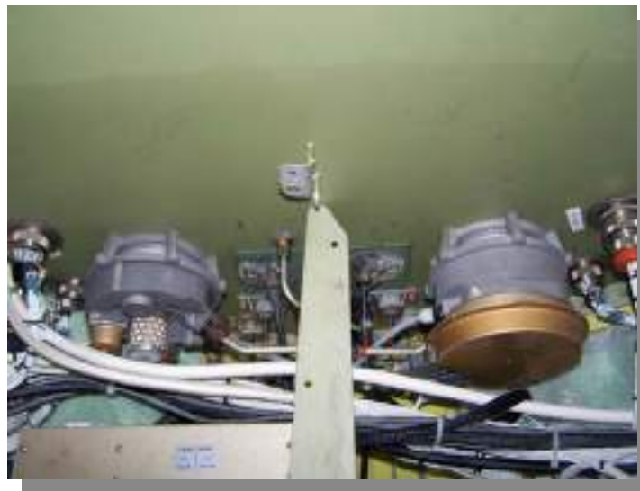
Figure 135. Secondary and Primary Outflow Valves
