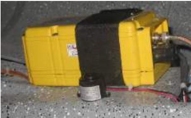
Fig. 7-24 ELT Artex ME406 installed
